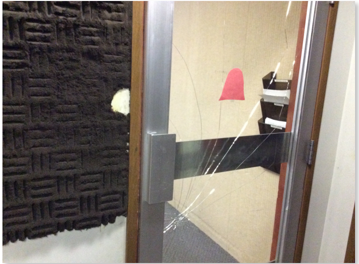
Deteriorating acoustic treatment and damaged door.
