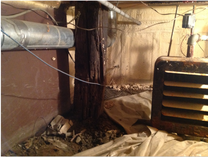
Rotting support posts under the VFCM headquarters.
